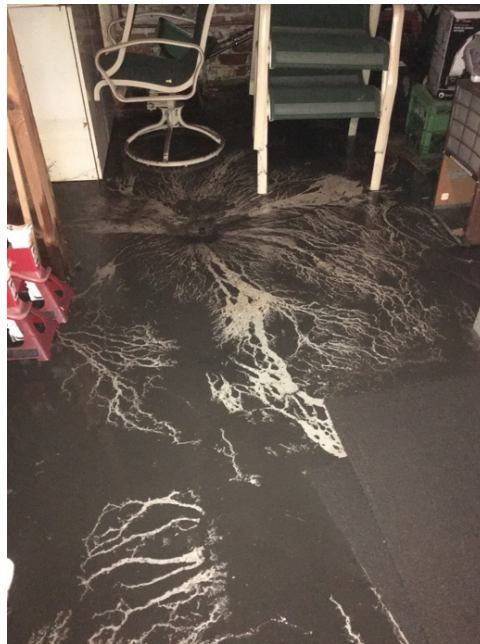
FIGURE 84: SEDIMENT IN BASEMENT
