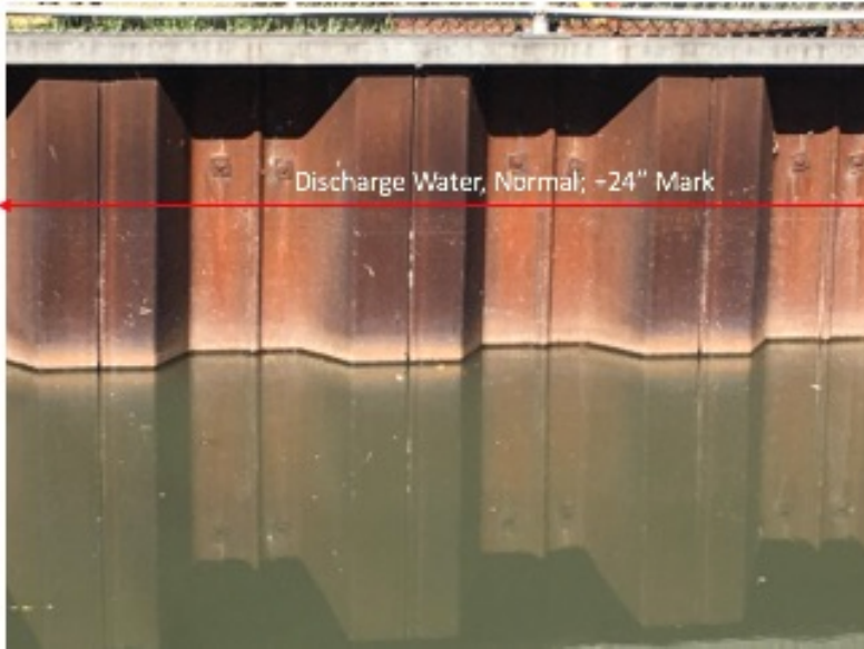
FIGURE 82: EVIDENCE OF WATER LEVEL 24" ABOVE NORMAL
